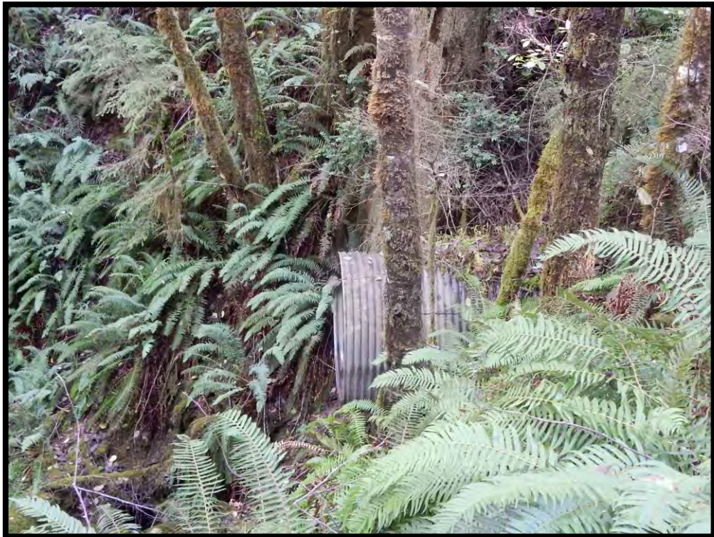
Figure 2: Photo Point #2- Class II shot gunned culvert on MM Road
