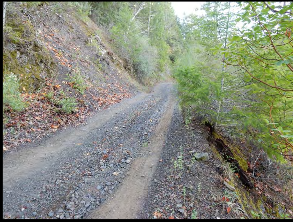
Figure 13: Photo Point #18- Slide on Reist Ranch Road
