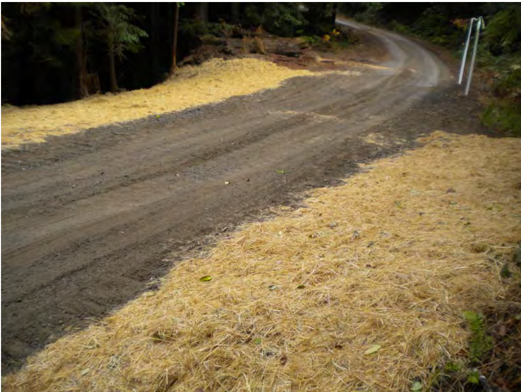
2012 Photo Point 4. M&M Road, upgraded road, rolling dip and cut off inboard ditch
